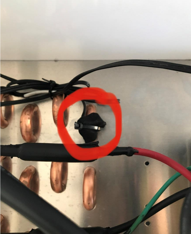
Unit cooler thermo sensor position-in air cooler right wiring box
