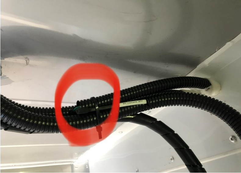
Return air thermo sensor position-back of air cooler right side
