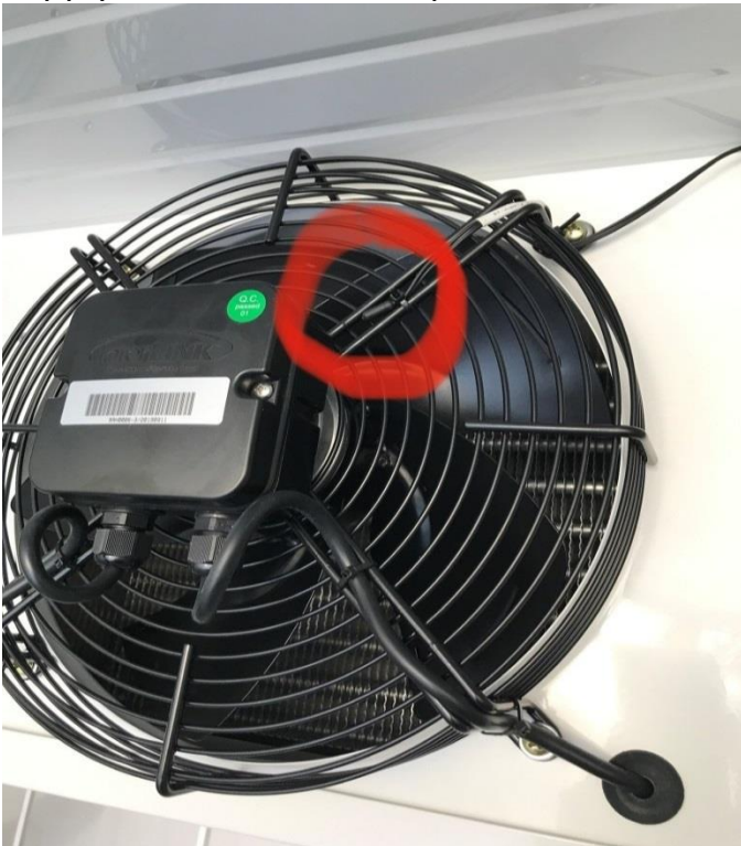
Supply air thermo sensor position-air cooler right fan
